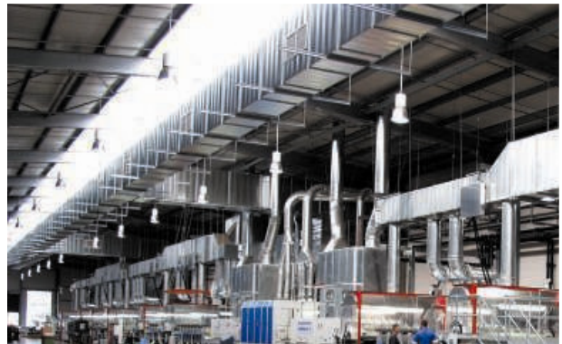
Figure 2: Factory Air Extraction for Mercury Vapour Lamp
